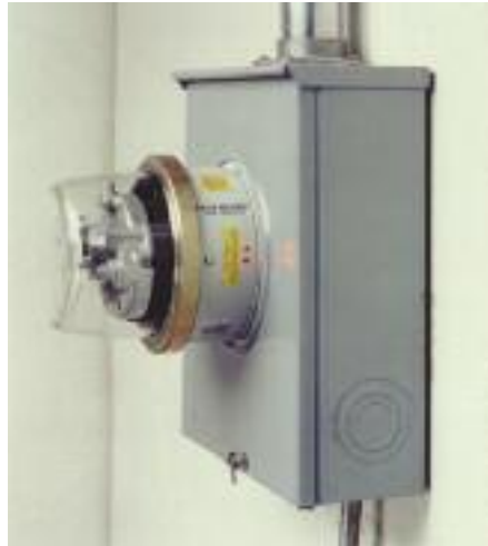
The electric meter is installed over the top of a base-type surge suppressor. It must be installed by an electrician. Photograph provided by Meter-Treater
