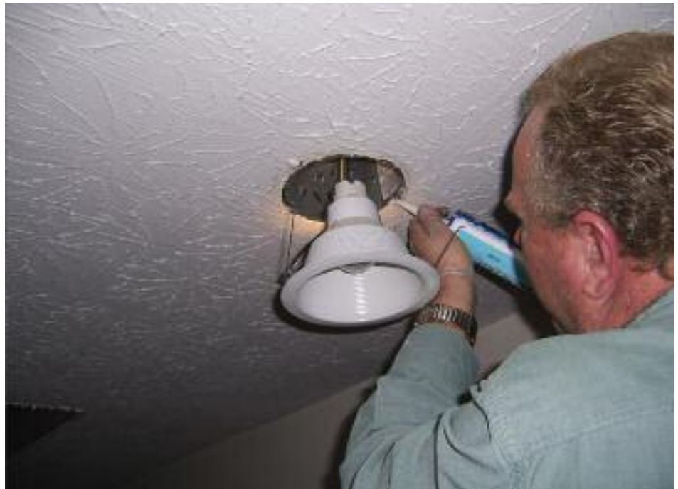
Sealing the cracks around recessed can lights with caulk can greatly reduce air flow. Photograph provided by Blue Grass Energy
